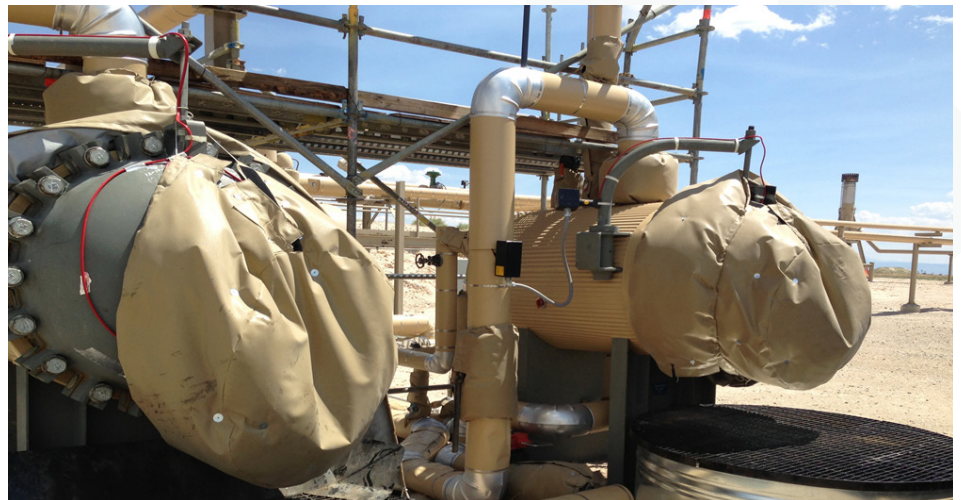
ProcessOR skidded vessels
