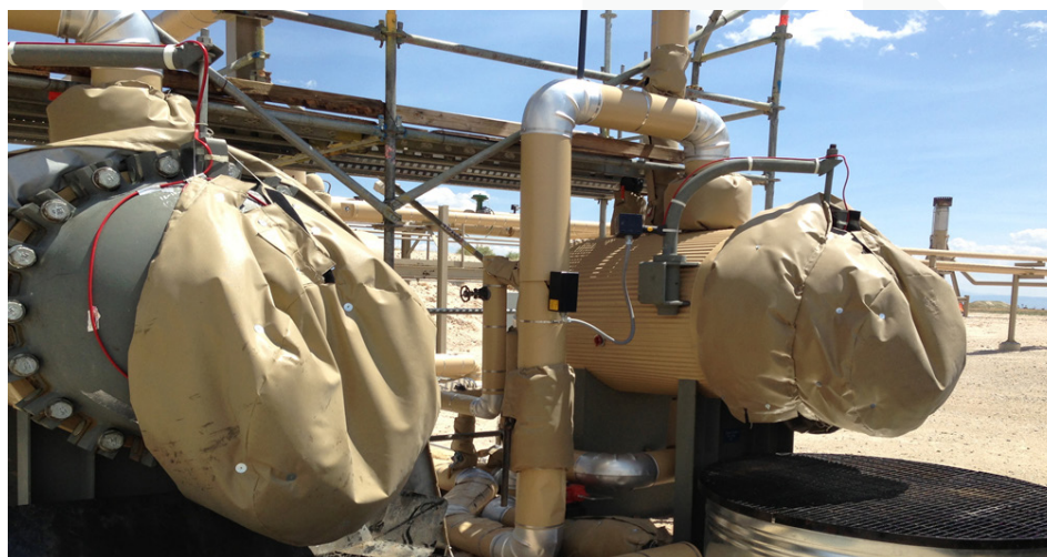
ProcessOR skidded vessels
